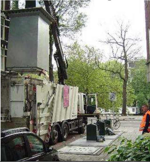
Recycling receptacles built into the sidewalk is an example of integrated city infrastructure and waste collection services.
